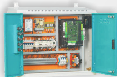
Close Loop Integrated Control Panel
