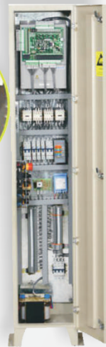
MRL Elevator Control Panel
